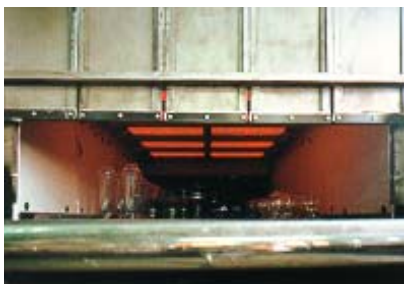
Metal fiber burner mounted in the roof of the annealing furnace for heating household glassware. (product temperature : 520 ~ 620 °C, burner surface temperature : 960 °C)
